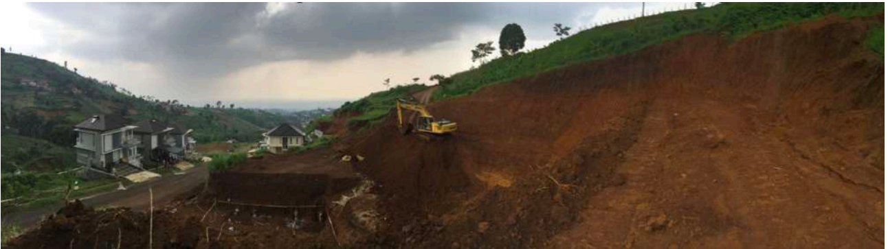
(Top left image) Site Research: Troy's (landowner's son) land, (top right image): I Made Ananta (Artist Assistant) with a Dago Pakar Resor construction worker, (bottom) Site Research: Dago Pakar Resor construction site
